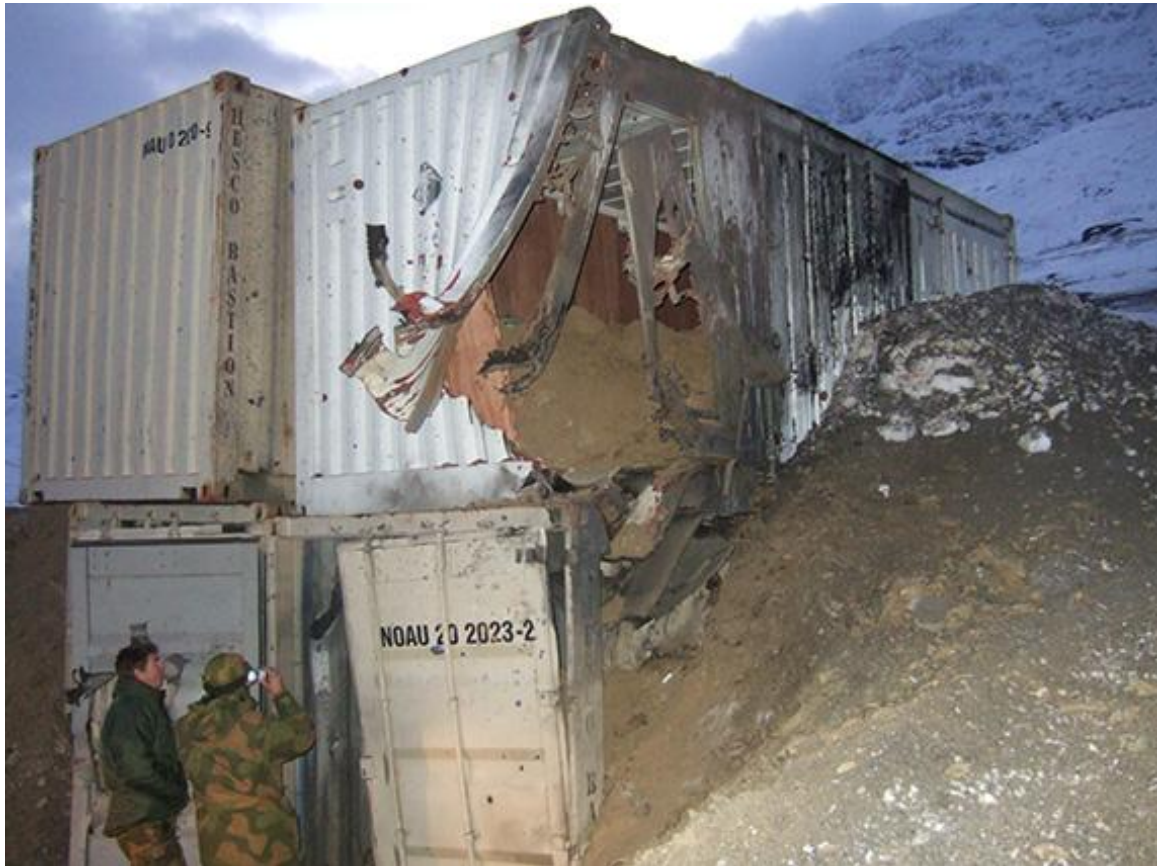
Figure 2.31 Results of a direct hit by a 155 shell at an INTOPS shelter
