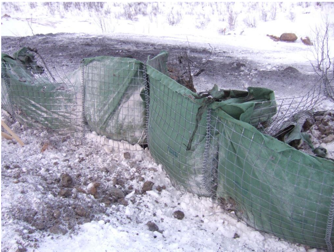
Figure 2.11 Back side of wall after test 1.3
