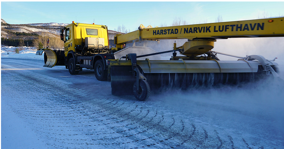
Figure 1.1 Sweeper truck performing maintenance on a frozen sand test field (curved lines on the ice) on a taxiway at Evenes Air Station. Photo: FFI.
